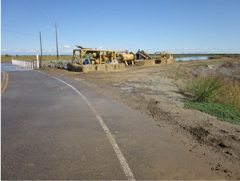
Photo 5: Pumps and compressors setup adjacent the Glenn Colusa Canal for hydrostatic testing of the pipeline.
