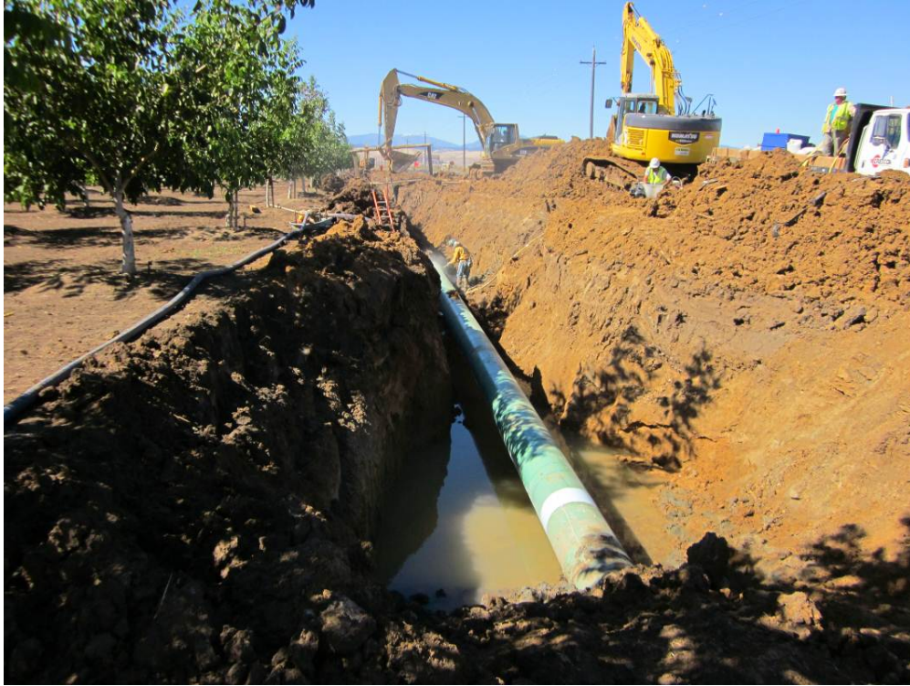
Photo 3: Pipe welding and backfilling of the trench along Dirks Road (between D-57 and D-59).
