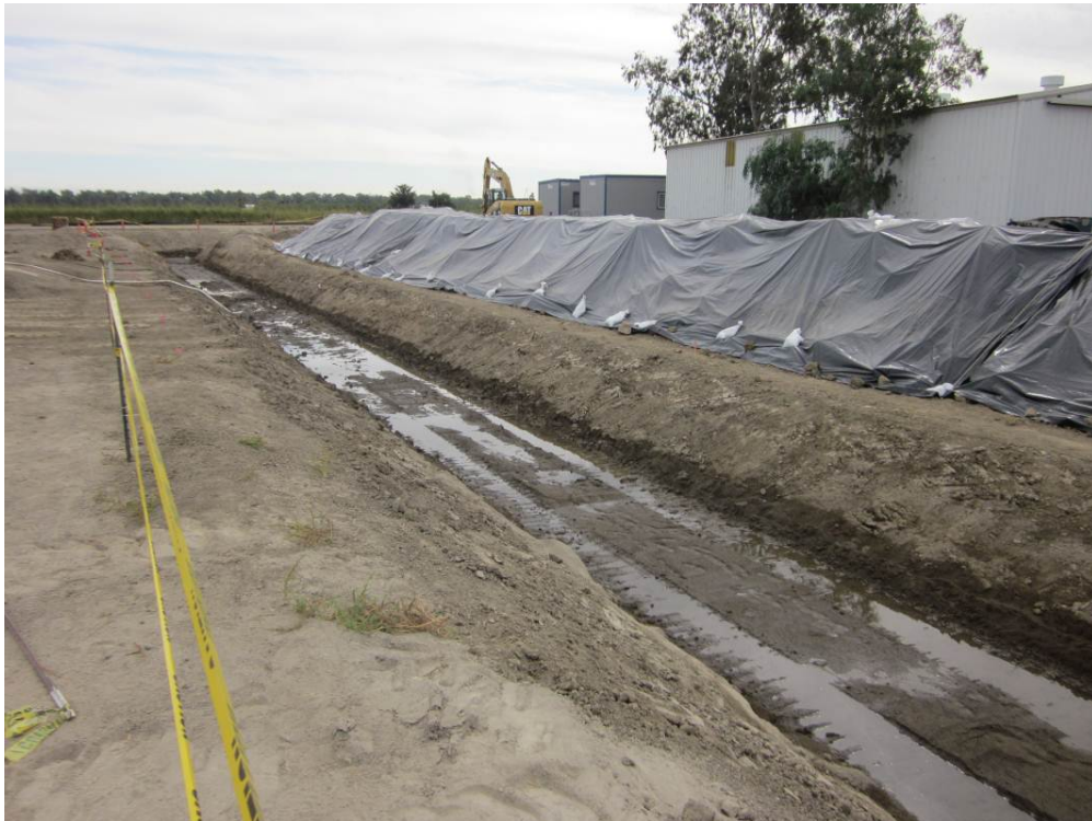
Photo 2: Excavated trench at the south end of the Compressor Station site. Excavated soil covered in anticipation of upcoming rain event.
