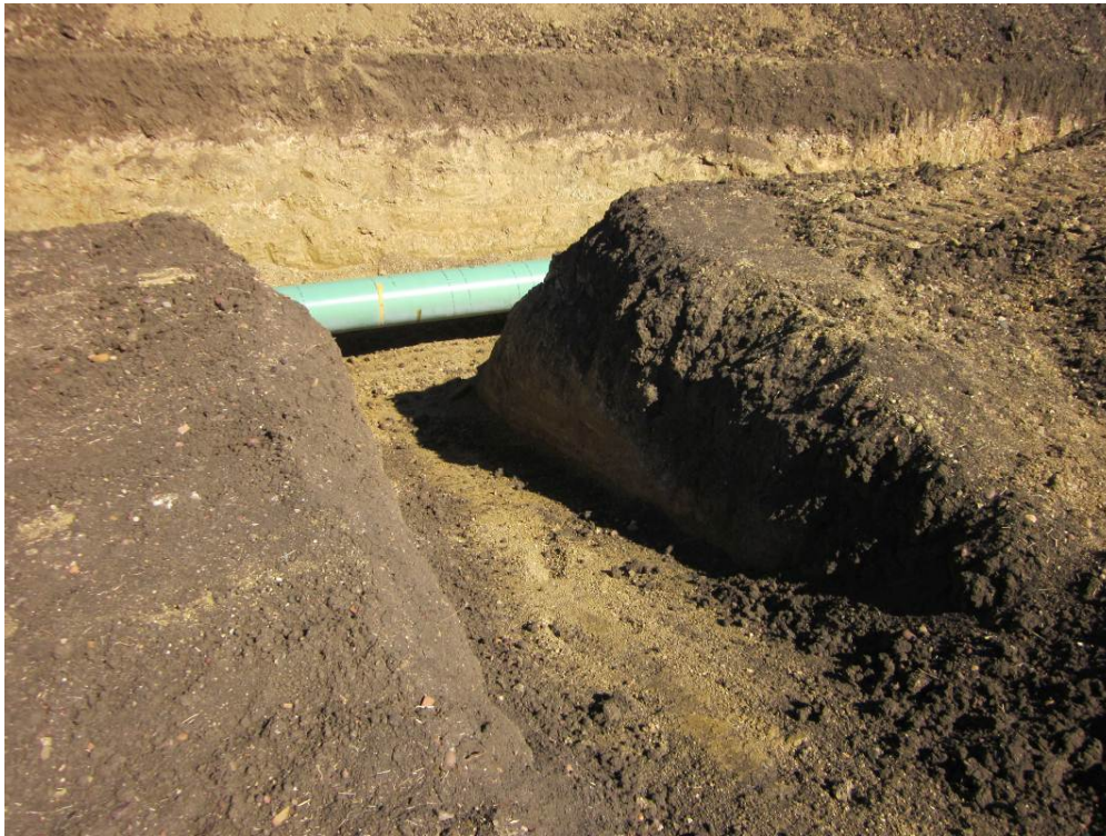
Photo 6: Pipe lowered within the trench between the Metering Station and the 400-401 Line Interconnect. Wildlife ramp installed along the trench to facilitate wildlife exit if necessary.
