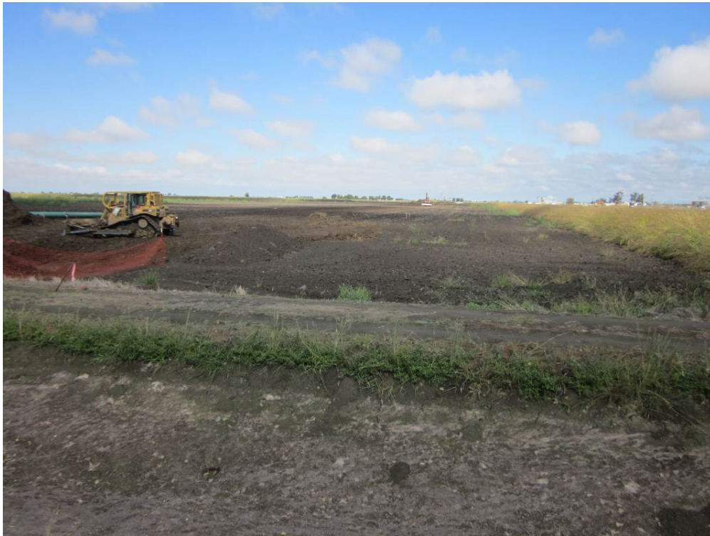
Photo 4: Trench backfilling and grading of the right-of-way between D-5/Dodge Road and the Remote Well Pad site.
